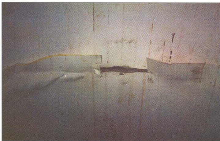
Liners historically have been used to prevent sewer manhole corrosion, although they can delaminate and wear thin over time. Any mistakes in installing them may render the liner useless.
