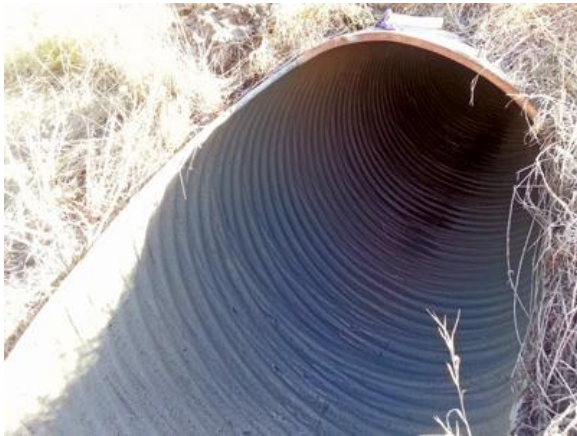
The Athabasca twin culverts were 48-in., cylindrical CMP culverts, running parallel beneath Highway 2, and about 33.5 m long.
