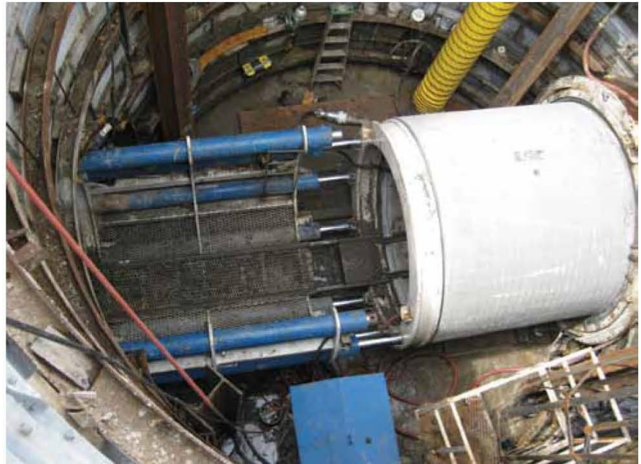
Concrete was selected because of its ability to withstand the jacking forces and depth of bury for this project.
