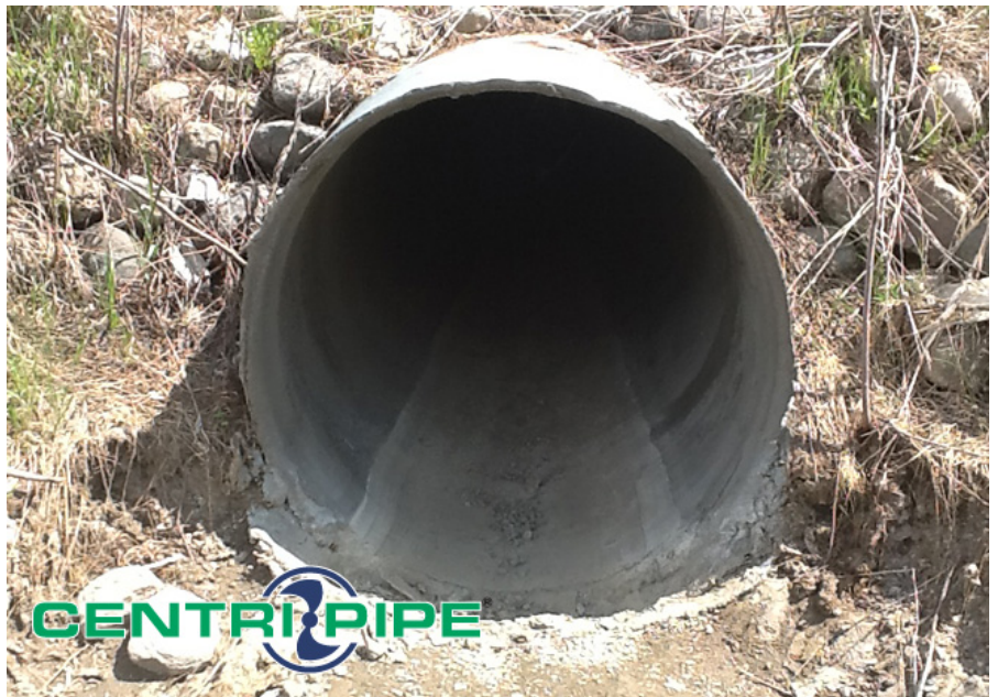
48" CMP culvert relined with centrifugally cast CentriPipe concrete liner. No significant reduction in flow capacity.
