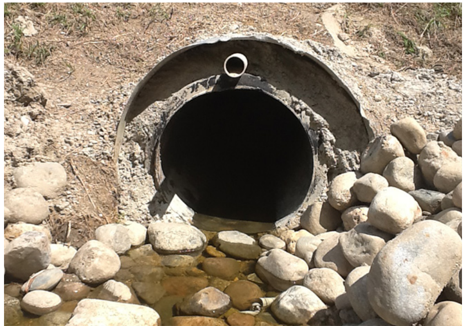
About half a kilometer up the road, this 48" culvert was rehabilitated with a slip-lining solution.
