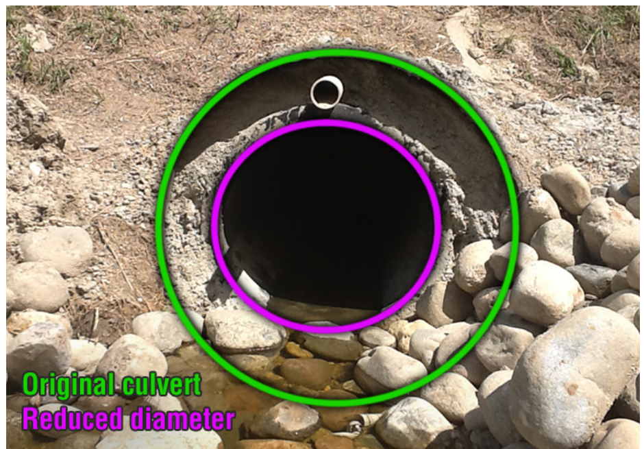
This culvert's ID was reduced from 48" to 30". The CentriPipe culvert's new ID is 46".
