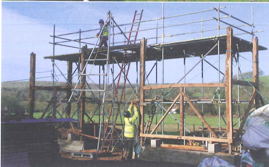
Work underway during the winter on the Eastwick Park Dairy, the Newdigate Bakehouse and May Day Farm barn.
