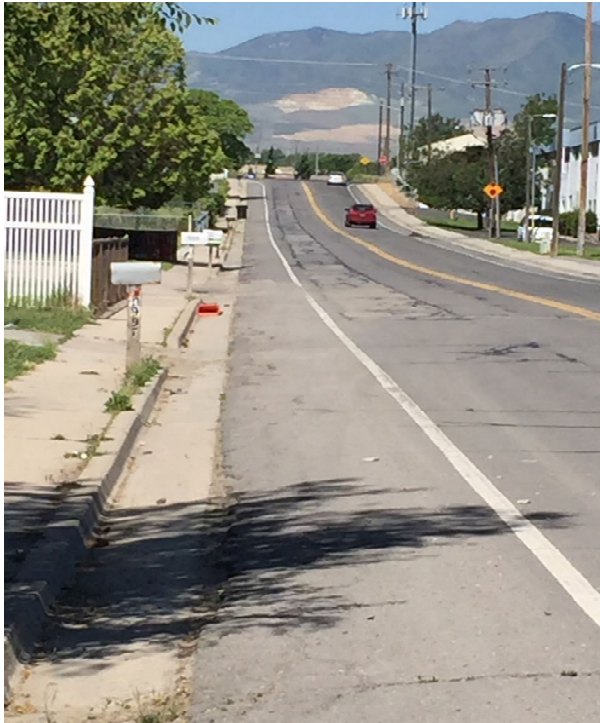
Existing shoulders in need of maintenance
