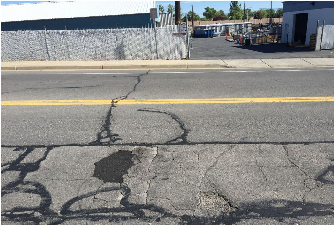
Existing Typical Asphalt Conditions
