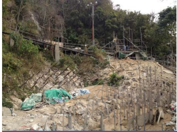
Installation of soil nails instead of mini piles to resolve the site constraint with limited space
