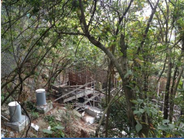
Construction of concrete baffle, concrete check dam and flexible barrier fence at steep terrain
